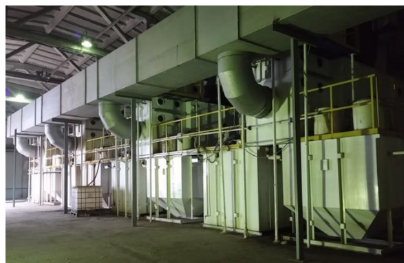
Figure 4 – The gas cleaning complex of four ABChUs with a total ventilating capacity of 100,000 m 3 per hour
